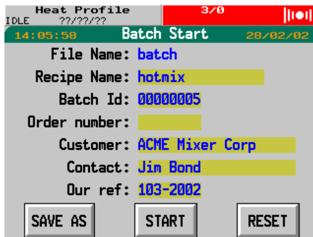
Figure 6-10 The customised Batch Start screen
